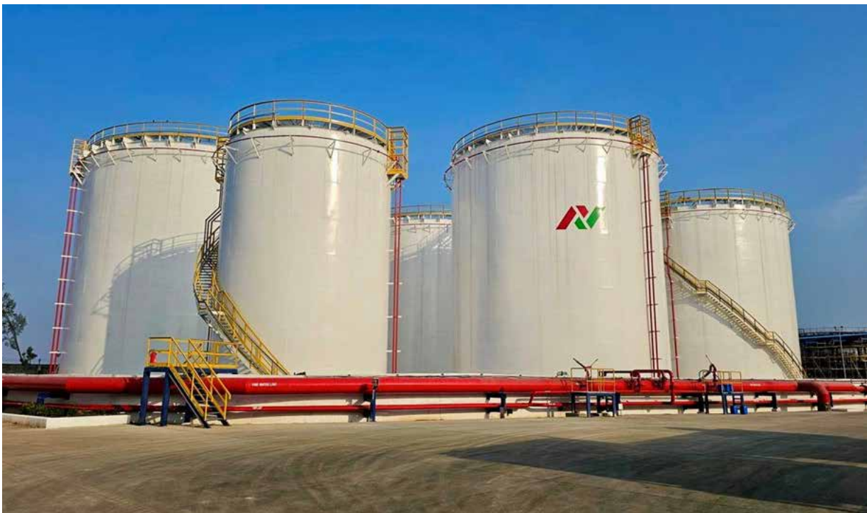
Newly commissioned liquid tanks at AVTL terminal in NMPT
