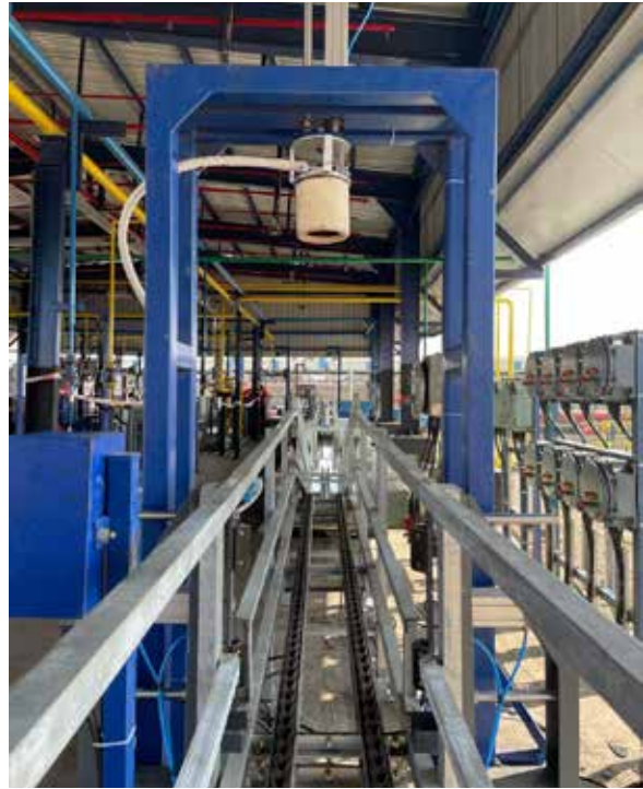
Newly commissioned LPG filling plant at Kandla LPG terminal
